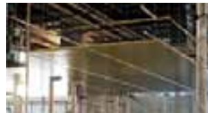
The 4 inch thick, stainless steel, walkable ceiling is cable-suspended from the [roof or steel frame] and withstands 27 psqf (pounds per square foot) to accommodate technicians and repair equipment.
