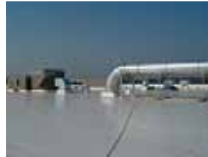
The white thermoplastic Polyolefin roof with heat-welded seams prohibits entry of bacteria-carrying insects and resists the effects of oily residue build-up emitted from the HVAC ventilation system during food processing.
